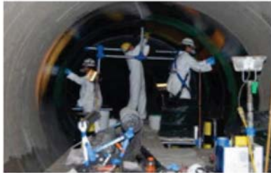
Prestressed Concrete Cylinder Pipe (PCCP) is widely used as water transmission lines: Components of PCCP, catastrophic failure of a 96-in. pipe, and retrofit of such pipes with wet layup carbon FRP application (2). StifPipe™ allows faster repair of PCCP at much lower costs than conventional CFRP liners shown here.
