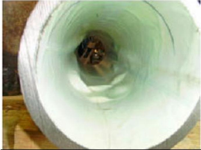
Figure 2-7 Liner Showing Installation Wrinkles
