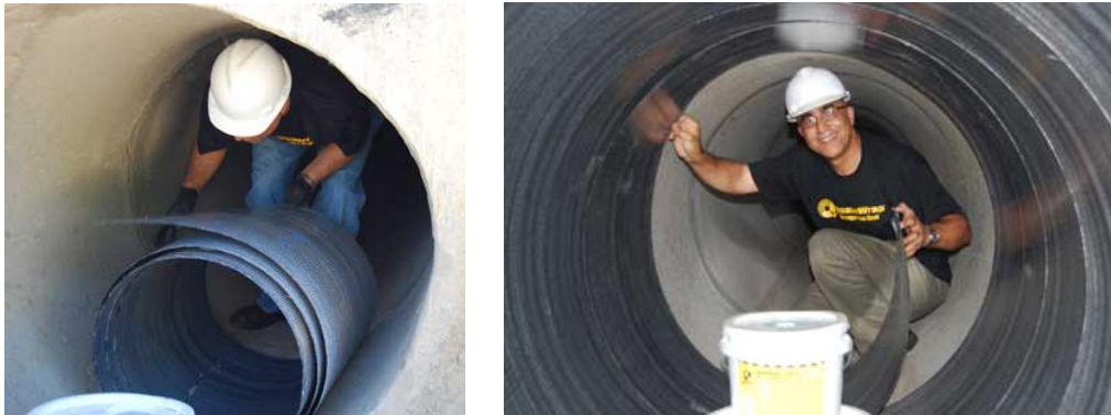
Fig. 3 – Super laminate being taken into the pipe and installed; one size fits all pipe diameters
