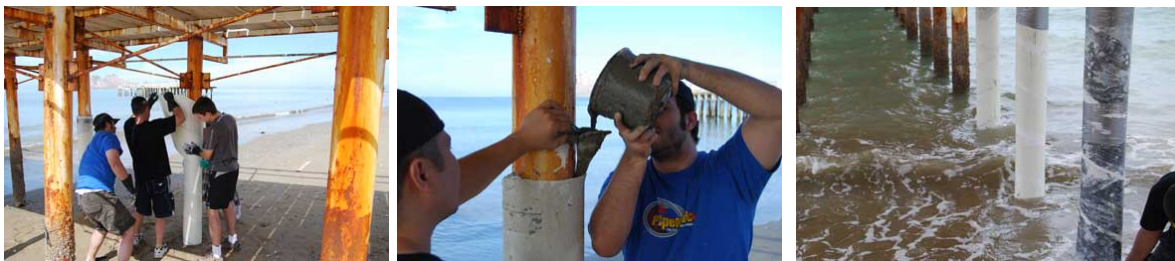
Fig. 7 – Retrofit of underwater piles; from left to right: construction of a seamless jacket with super laminates; filling the annular space; completed pile jacket
